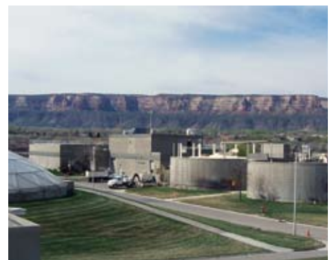
Energy efficiency improvements at the Persigo Wastewater Treatment Plant will yield over $23,000 in utility savings annually.
