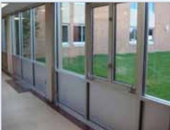
Western's original windows leaked and did not lock. Ameresco installed new heavier grade windows, which sealed the buildings and improved occupant safety.
