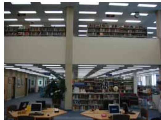
At Savage Library, Ameresco re-commissioned the air handlers and performed a lighting retrofit to improve the air quality and study space.
